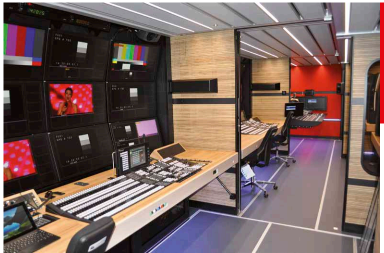
Figure 1: Video control room A and B, and audio control room A
